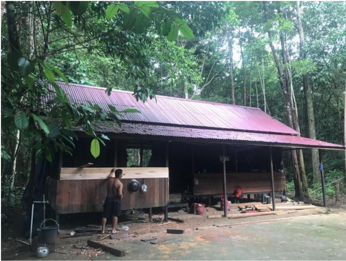
Repairs being made to the building at the Rangkong camp in preparation for full capacity research data collection there.
