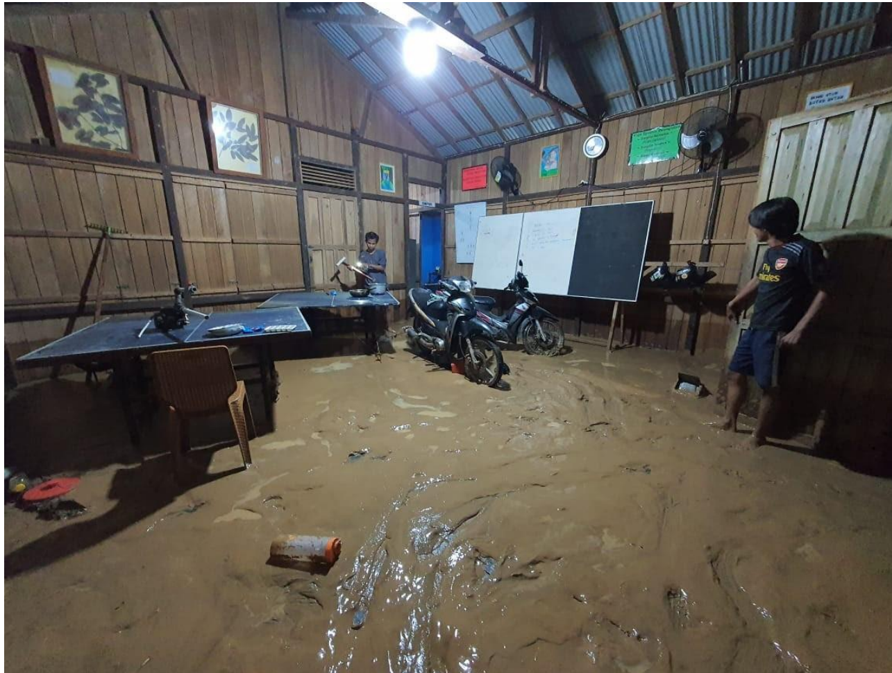
Mud covers the floor inside Bentangor the day after the building flooded.
